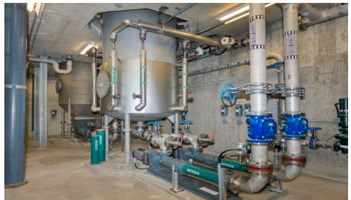
Pictured: Inside the Facility.
