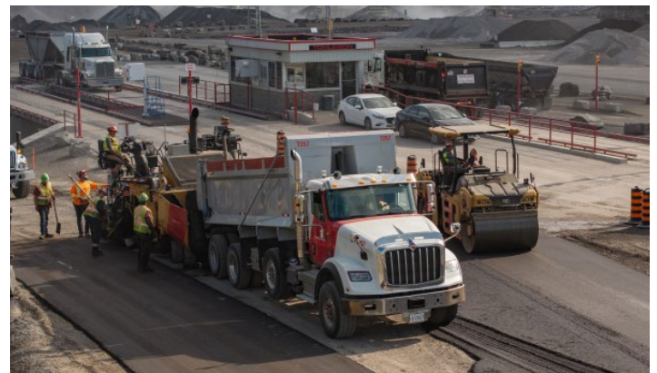
Pictured: Laying of Low CI Asphalt Mix on scales pathway at Rideau Quarry.
