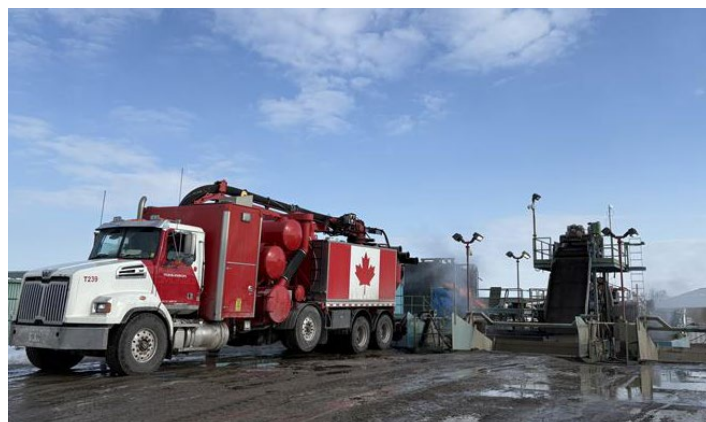
Pictured: Tomlinson VAC Truck emptying the debris tank at Bantree Reclamation Facility.
