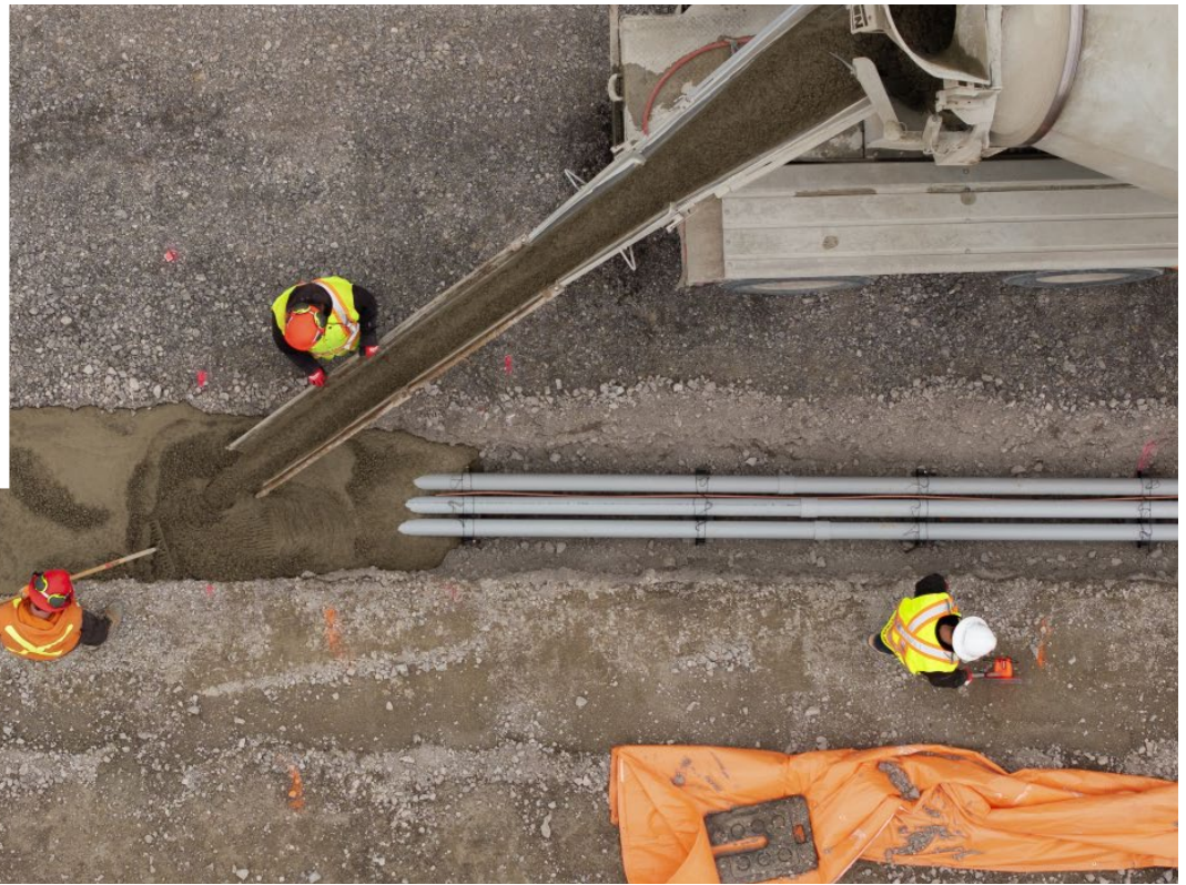
Pictured: Tomlinson Ready Mix backfilling conduit and duct banks with thermal lean concrete fill to dissipate heat from electrical lines.
